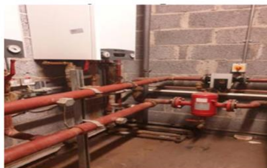
Plantroom Boiler & pipe works
